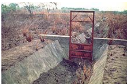
Fig. 2. Drainage infrastructure in what was a plantation of Gros Michel in Honduras. Before 1960, widespread destruction of Gros Michel was common in export-producing areas in tropical America and western Africa (courtesy of Phillip Rowe) (click image for larger view ).
